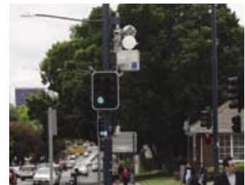
In the city of Liverpool, Australia, PASOLINK has been adopted as the data transmission infrastructure for surveillance cameras and other systems.
